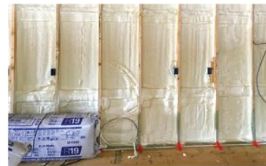
Blown fiberglass packs the wall cavities, which are first air sealed with an inch-thick coating of open-cell spray foam.
